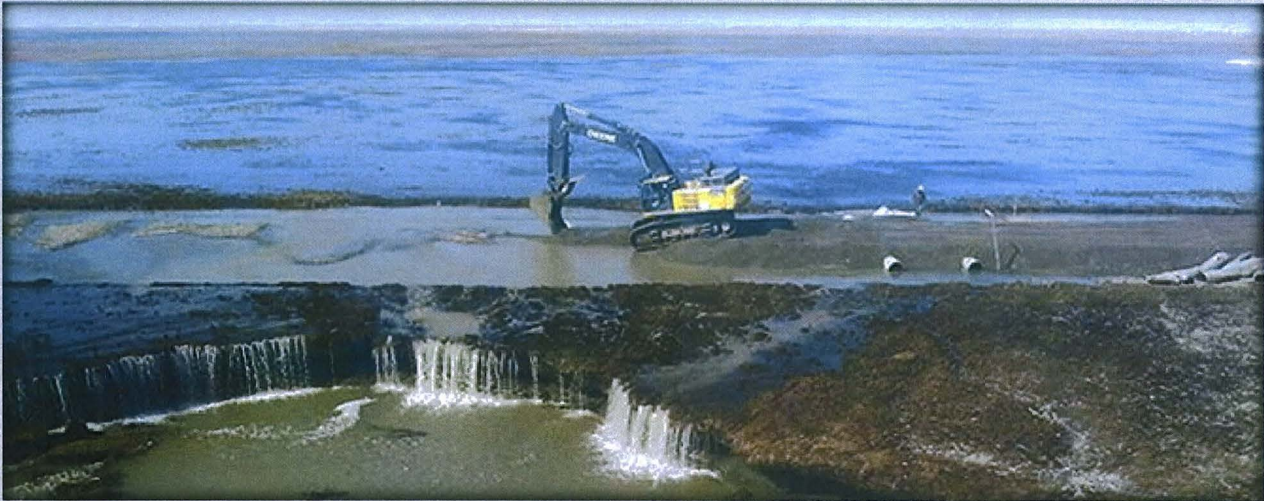
DOT&PF M&O repairing Dalton Highway during excessive spring flooding, 2015. Photo by Alaska DOT&PF
