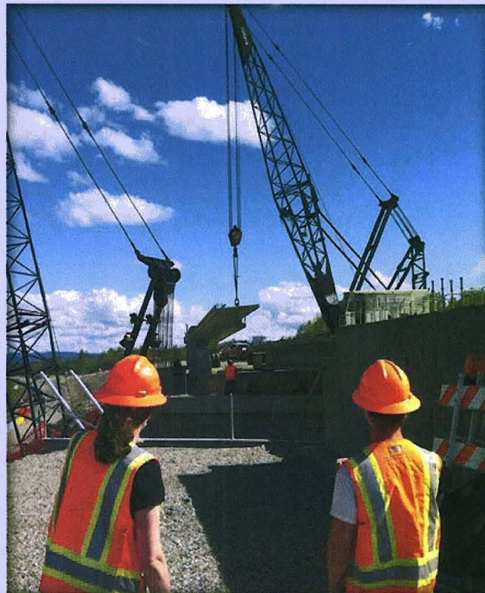
Bridge Section's Leslie Daugherty and Will Strehler observe as cranes pick up a girder of the Moose Creek Railroad Bridge. Photo by John Orbistondo, Alaska DOT&PF
