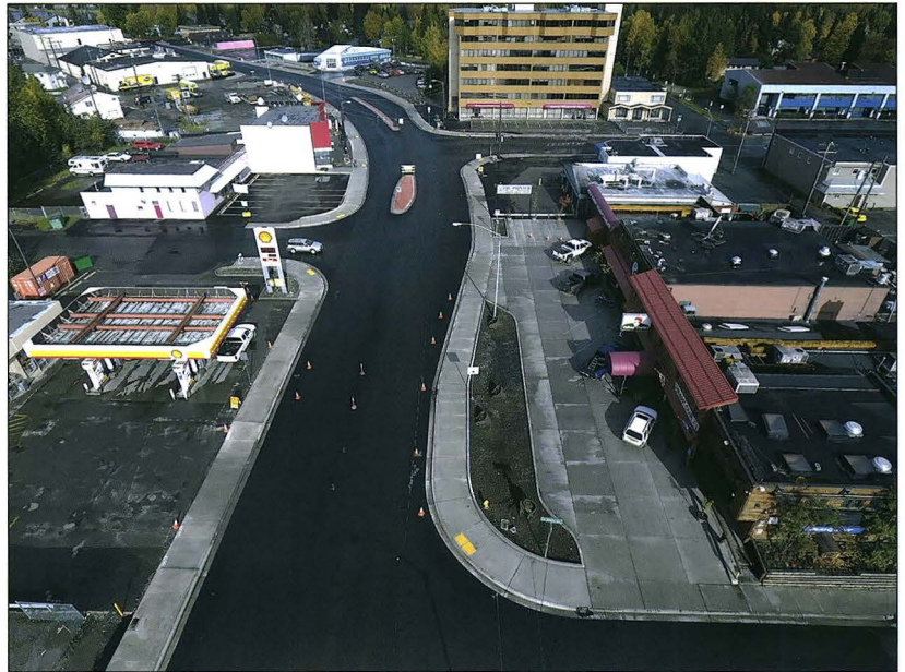
SPENARD ROAD RECONSTRUCTION PHASE II, QAP
