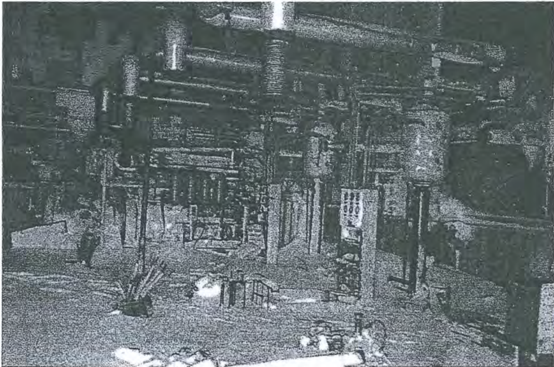
Figure 9. Transformers Containing PCB's at Driftwood Bay (ANCSA selected, not conveyed)
