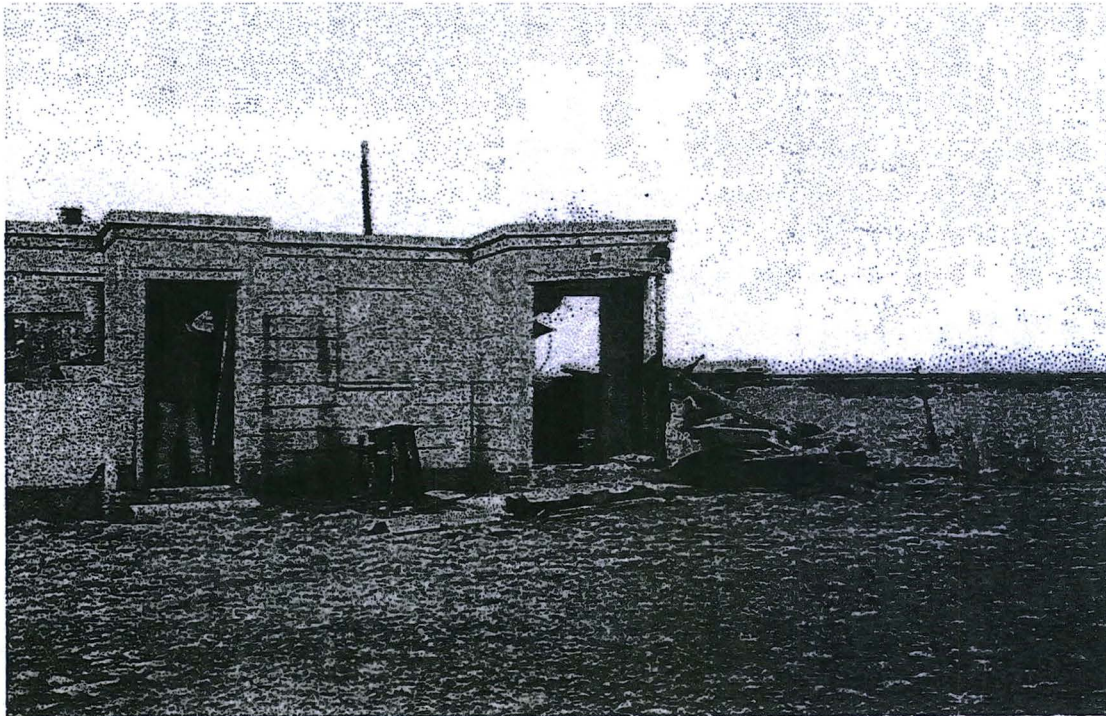
Figure 11. Former FAA Site at Middleton Island Known to Contain Asbestos
