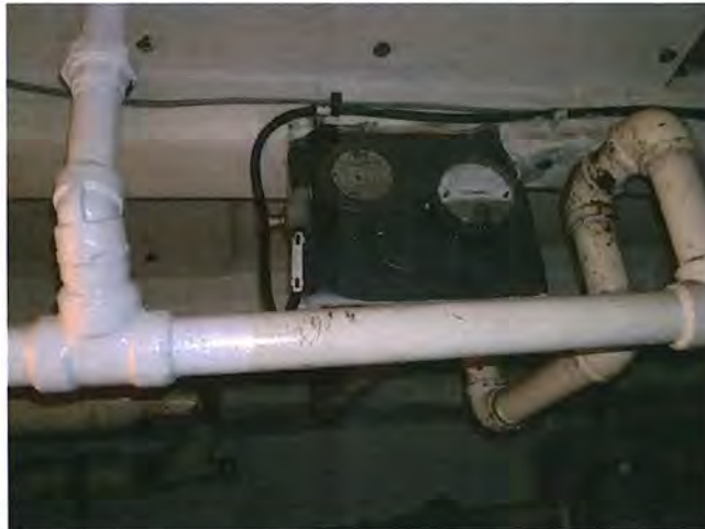
Photo 6-4 : Non Operational Port Vacuum Sensor and Gauge
