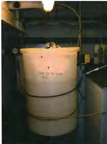
Photo 6-1 : External Chlorine Injection Tank
