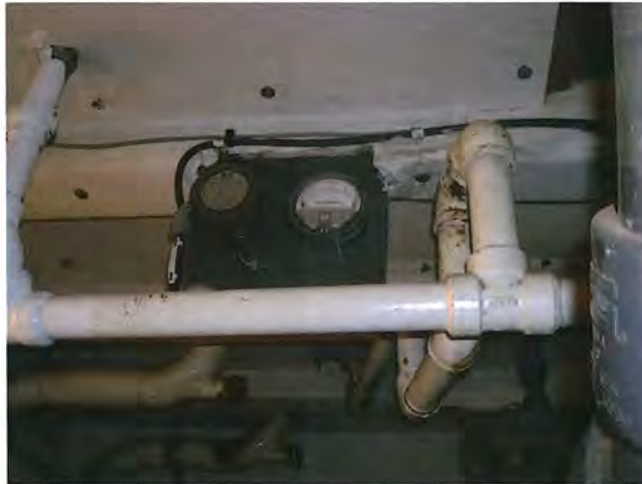
Photo 6-3: Non Operational Center Vacuum Sensor and Gauge
