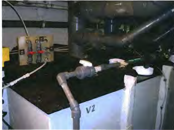
Photo 6-2 : External Chlorine Injection Distribution Manifold
