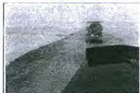
Overflow on Alaska's Dalton Highway
