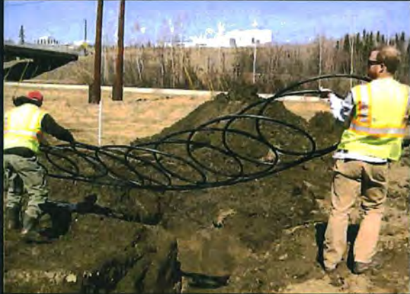
Fairbanks Ground Source Heat
