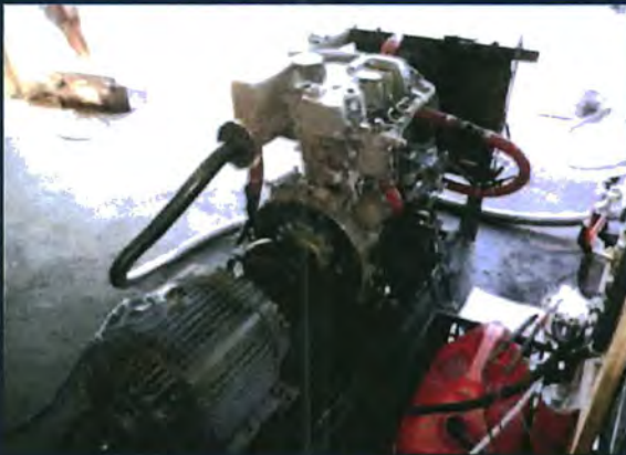
Modified 15 kW genset
