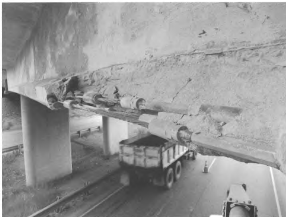
Figure 13. Highway Overpass Damaged by a Vehicle Collision
