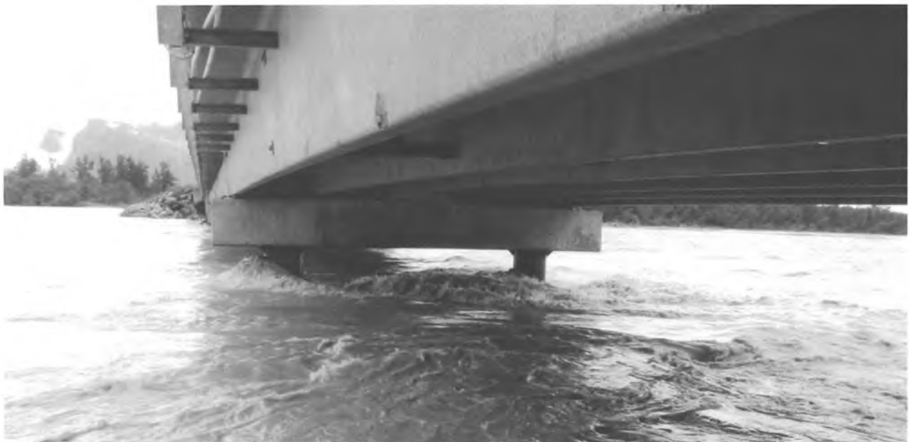
Figure 8. Active Scour on Bridge #339, Copper River Highway
