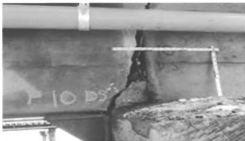
Figure 6. Deteriorating Concrete Trail River Bridge
