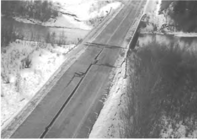
Figure 9: Earthquake Damage on the Richardson Highway
