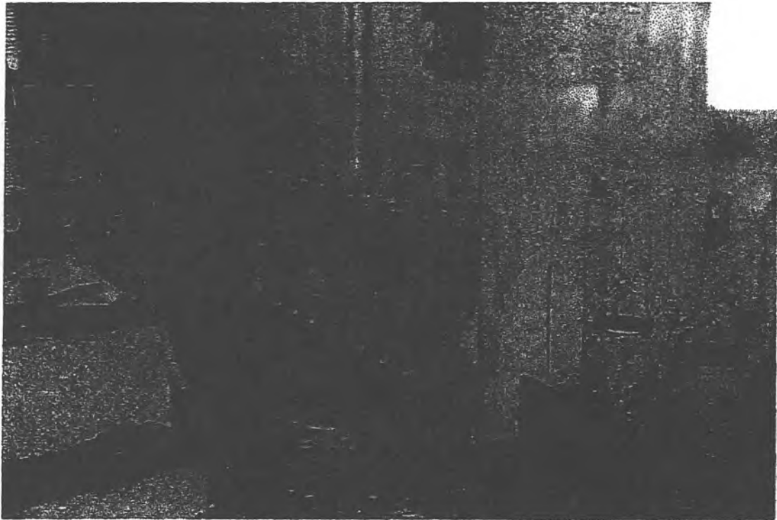
Figure 8. Batteries inside Building (since removed) at Middleton Island
