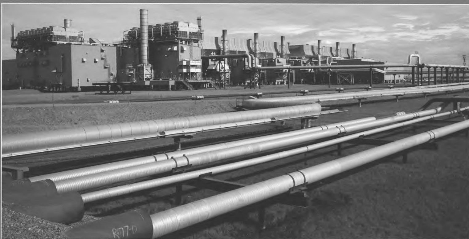
Central Compressor Plant at Prudhoe Bay
