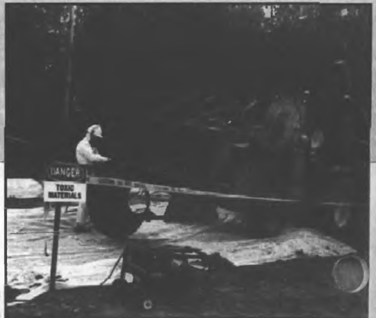
A worker at a cleanup operation dressed in "Level C" protective gear.
