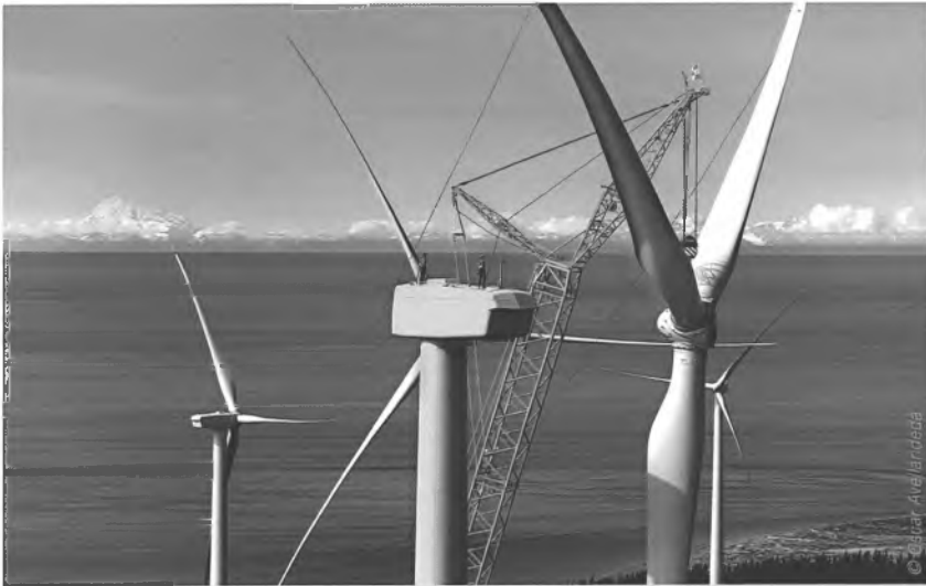
CIRI's Fire Island Wind turbines
