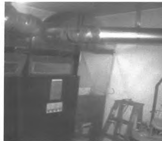
Sitka Public Health Furnace Replacement After
