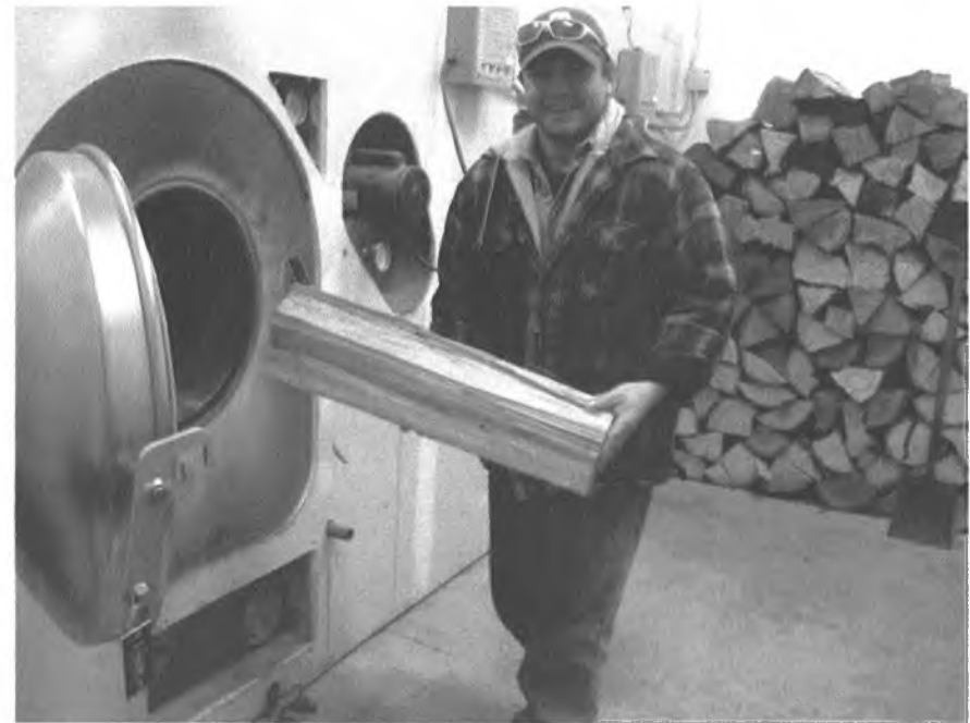
Coffman Cove School Garn boiler.
