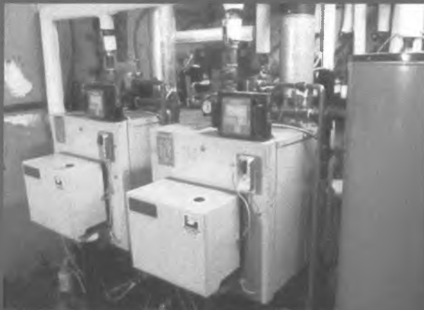
Emmonak City Hall boiler before and after efficiency improvements
