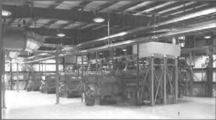
GE Jenbacher gas engines at Doyon Utility's JBER facility
