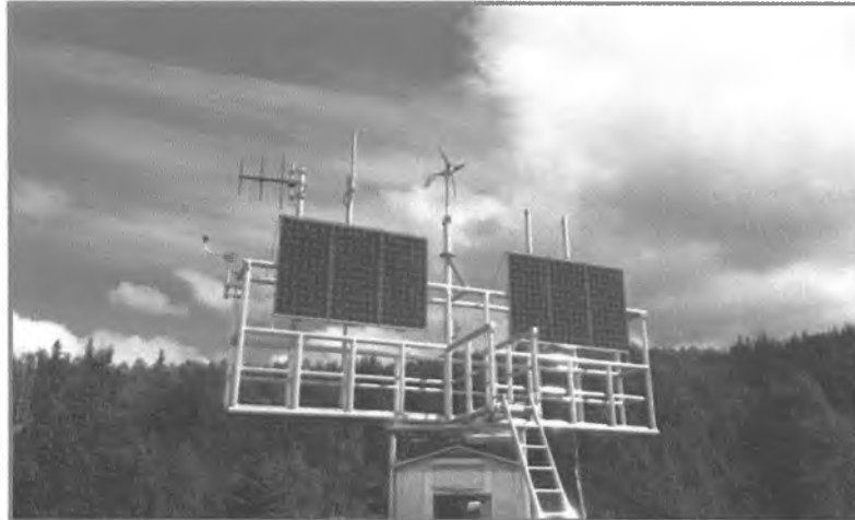
PTC wayside switch monitoring at Potter siding with antennas for GPS, train to wayside data radio, and office to field data radio. Note solar and wind power generation.
