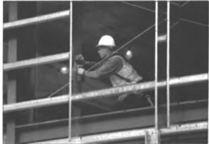
Floyd Frank screws a bracket into the metal framing Wednesday at KIC's new facility currently under construction at the corner of Stedman and Deermount Streets.
