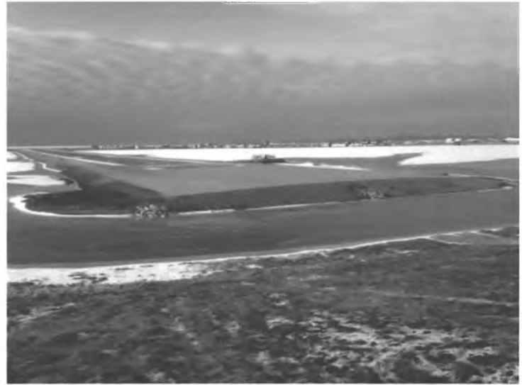
Kotzebue Airport - view of new runway safety area constructed on runway east end.
