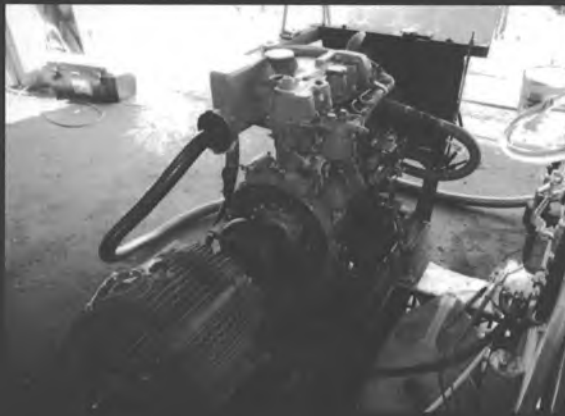
Modified 15 kW Genset
