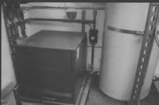
Installed 3-ton Heat Pump
