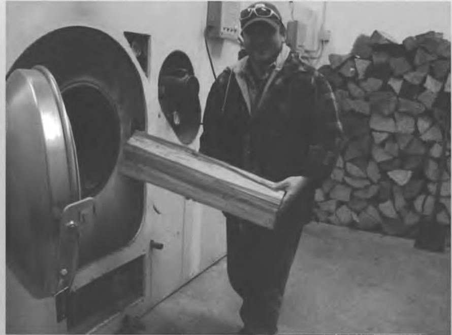
Coffman Cove School Garn boiler.
