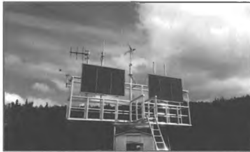
PTC wayside switch monitoring at Potter siding with antennas for GPS, train to wayside data radio, and office to field data radio. Note solar and wind power generation.
