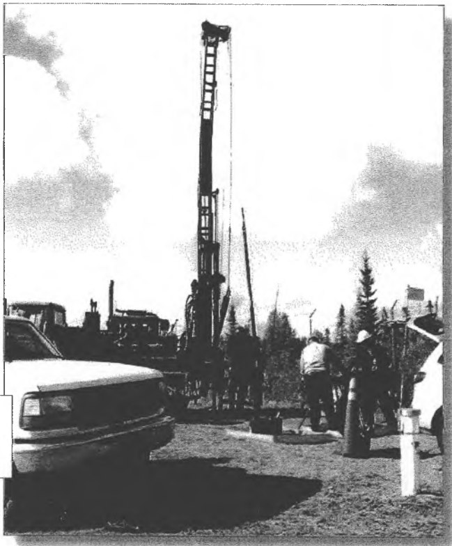
(Right) A Flint Hills contractor drills into the ground to install a new monitoring well, one of 80 installed this summer. (FHRA photo)
