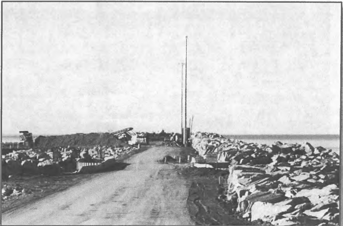
Photo 4 Completed High Mast Lighting
