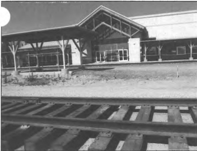
A second track is constructed parallel to the existing track by the Fairbanks Depot.
