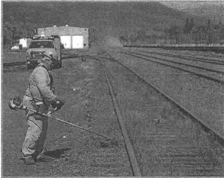
Manual vegetation control (weed trimming/mowing) In the Seward Yard is not adequate or lasting.
