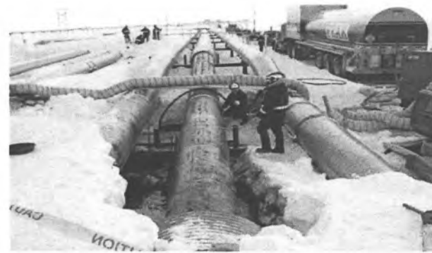
GC 2 Pipeline Spill
