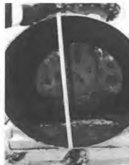
Sludge buildup prevented corrosion detection equipment from working
