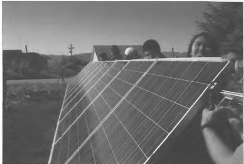
Angoon residents install a solar power panel on a home as part of the Sustain Angoon Project. Photo courtesy of Central Council, Tlingit and Haida Tribes of Alaska.
