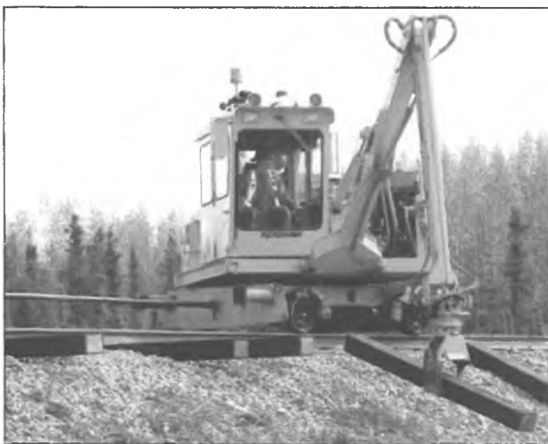
A tie crane operator positions a new tie during tie replacement operations in spring 2011.
