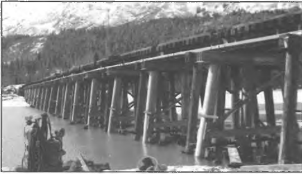
Timber piling and caps were replaced with steel pipe and pile caps on the bridge at MP 29.5 in 2011. In 2012, timber beams and ties will be replaced to complete bridge rehabilitation.
