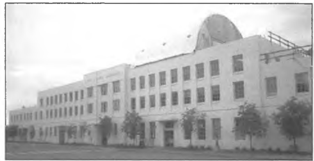
Phase 2a included installation of a paved-system roof along with more insulation for better energy conservation.
