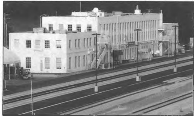
Phase One of the Ship Creek ITC constructs two new tracks and a pedestrian platform next to the Anchorage Historic Depot.
