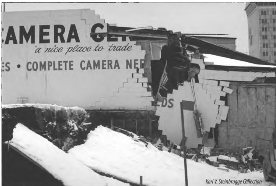
An un-reinforced masonry building in Anchorage collapsed during the 1964 Good Friday earthquake.
