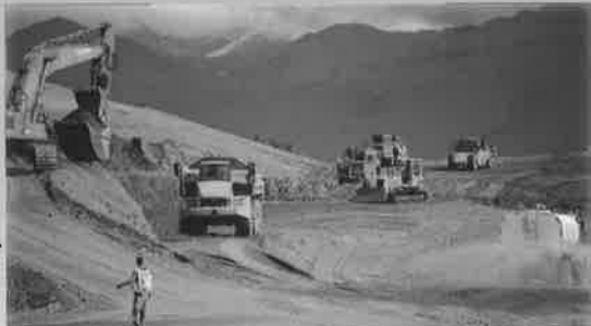
Photos: the ship, the deepest draft vessel ever in Upper Cook Inlet at Port MacKenzie; Above: 2010 haul road and rail loop construction at Port Mac moved 1.9 million cubic yards of dirt.
