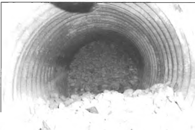
A culvert becomes clogged with ballast (track bed rock) leaking in.
