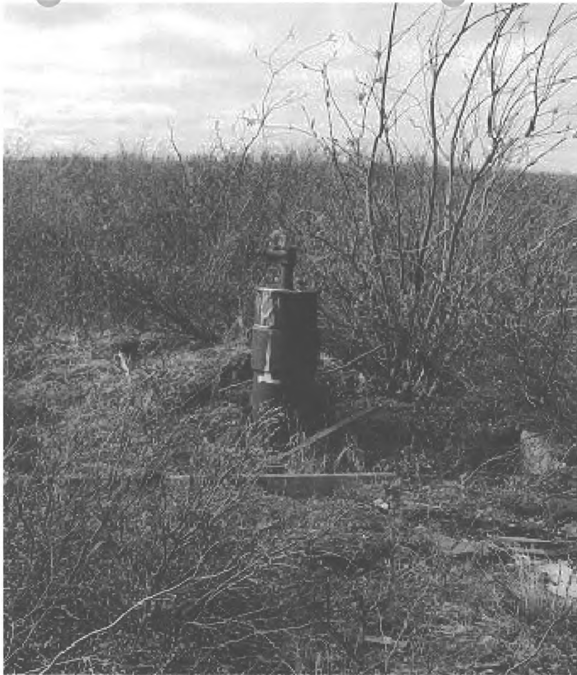
Primitive, rusting wellhead and wood debris
