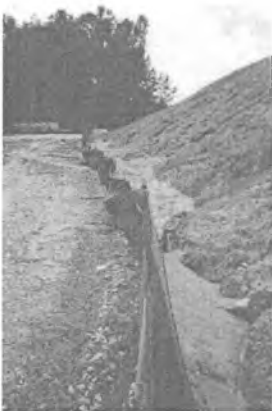
Sediment accumulation at a construction site.
