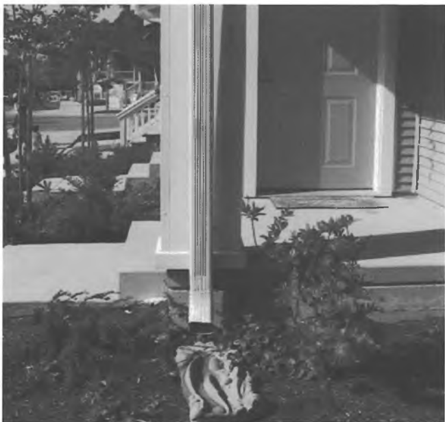
Downspouts that are not connected to the sewer system allow stormwater to be absorbed into landscaped areas.
