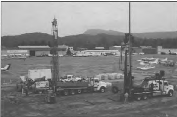
Figure 1. Vertical borings for JNU Airport loop field. Image courtesy of JNU staff
