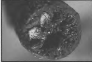
Zebra mussels blocking a pipe
