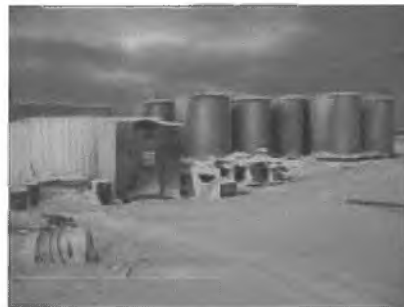
Rural Alaska fuel storage tanks
