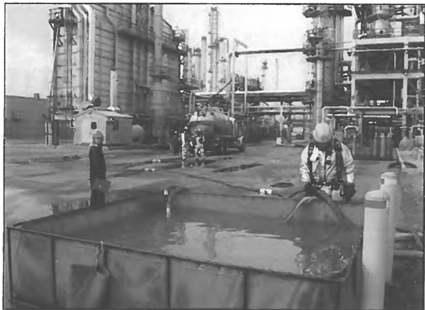
Ann Farris, DEC's project manager, is shown inspecting pumping operations. (DEC photo)
