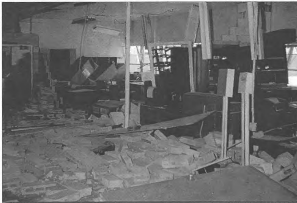
Shaking damage in the U.S. Weather Bureau office at Anchorage International Airport during the 1964 earthquake. Note the failure of unreinforced concrete masonry unit (CMU) walls and extensive nonstructural damage. Photo by A.L. Comiskey.
