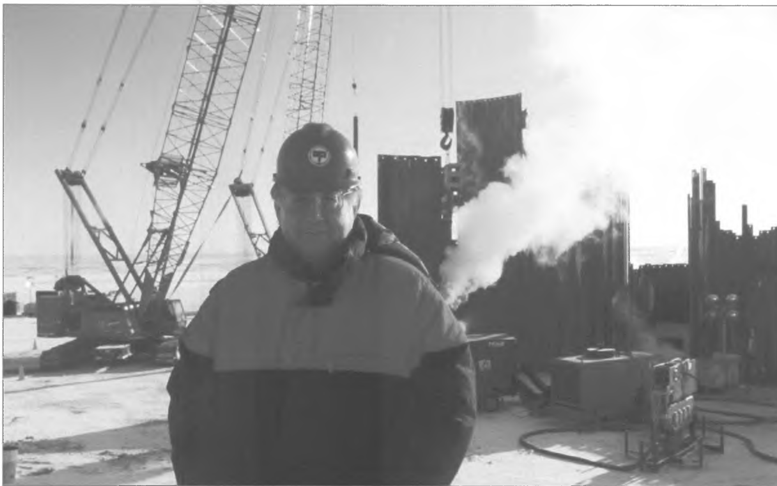
PND co-founder Dennis Nottingham on-site of OPEN CELL construction at Northstar Island
