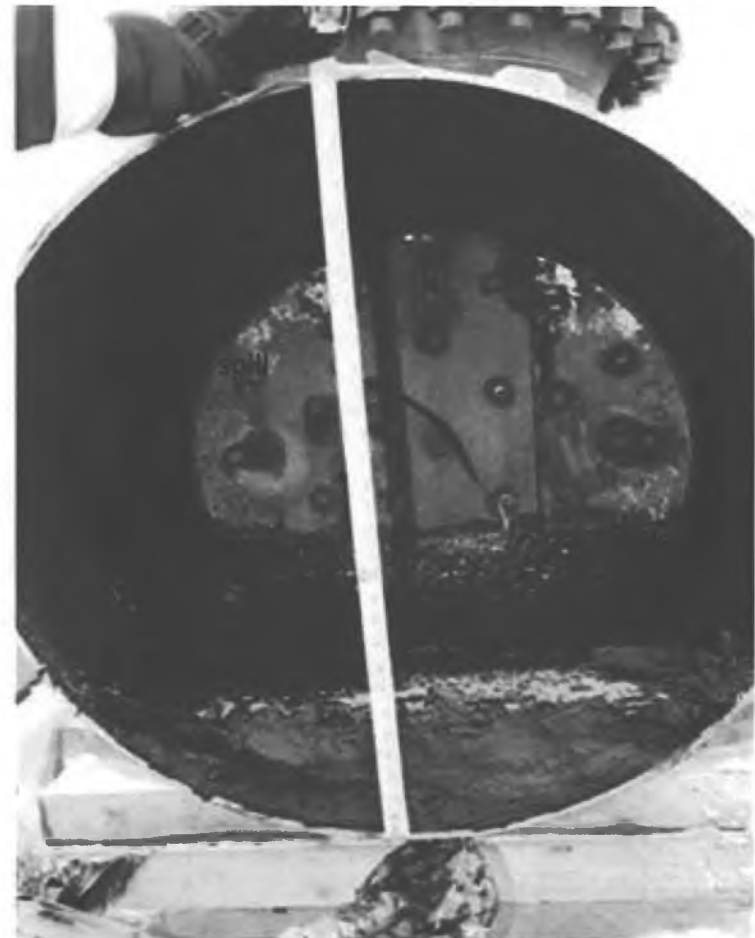
Sludge buildup prevented corrosion detection equipment from working
