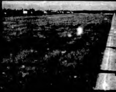
Birchwood Airport, pavement cracking
