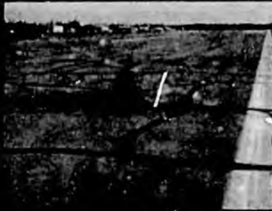
Birchwood Airport, pavement cracking
