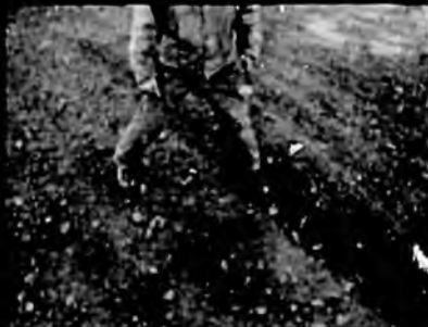
Savoonga Airport, runway rutting
