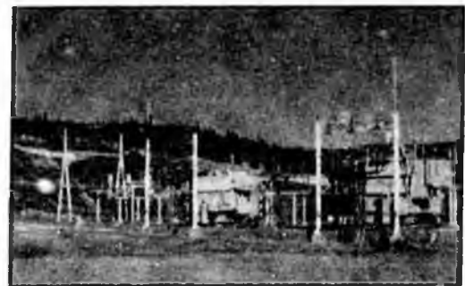
The electrical substation at Fort Knox is located near the mill building.
