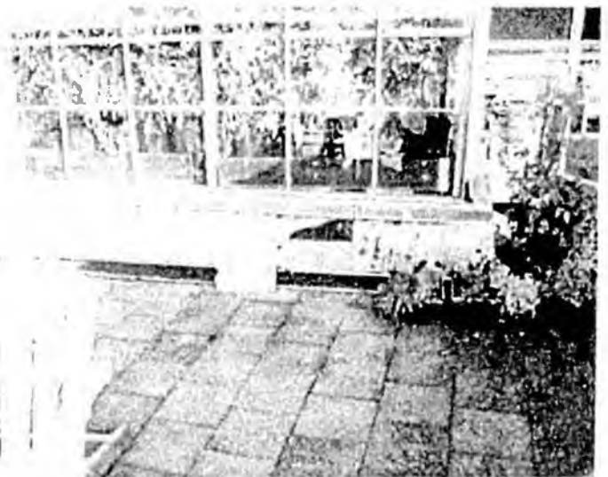
4. Deteriorated siding on wall area below greenhouse structure, Leak #1 is several feet to left of this area
