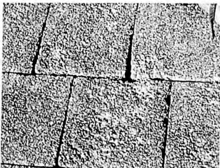
15. Erosion of the ballast pavers
