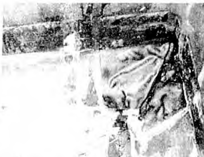
18. View of membrane flashing at Leak #2, EPDM should be smooth, water was found under this patch
