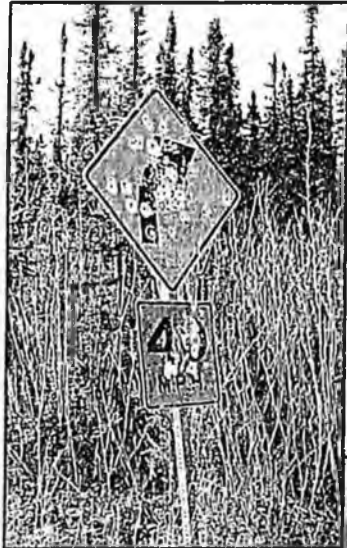
Above: Typical sign damage along an Alaska highway
