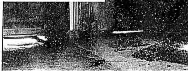
Right: Foundation and floor settlement at Chandalar Maintenance Facility
