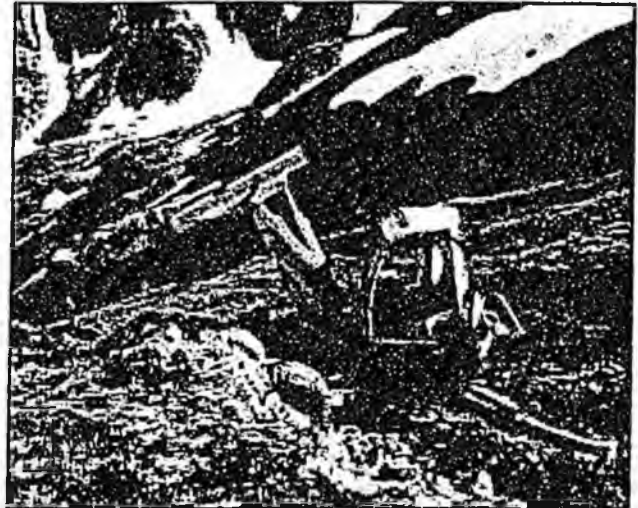
A "Menzi muck" machine carves out a trench to bury power lines. Photo is courtesy of Alaska Electric Light & Power Company.
