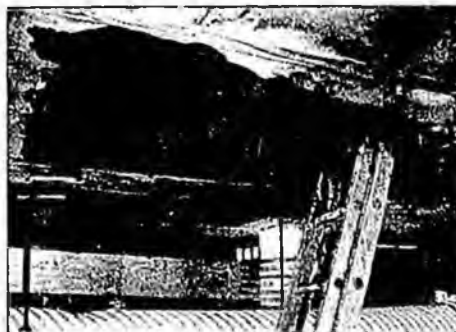
Schools In Peril Hooper Bay High School, Lower Yukon, shows rotted structural members. Extensive deterioration was discovered in the area of the bathrooms and showers during an appraisal in February 2001 by SERRC, Inc.
