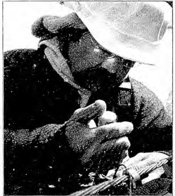
An Arctic Slope Telephone Association Cooperative, Inc. (ASTAC) telephone technician splices wires. Photo is courtesy of ASTAC.
