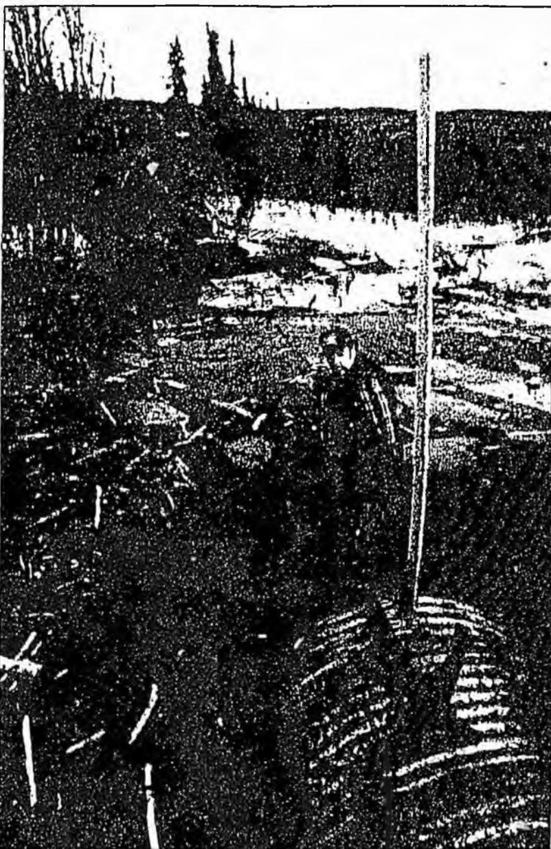
CLEARING CULVERT —Chuck Nichols, a worker for the Alaska Department of Transportation, prepares to insert a grappeling hook into a culvert at 3 Mile Chena Hot Springs Road on Tuesday to clear out the dam built by beavers.
