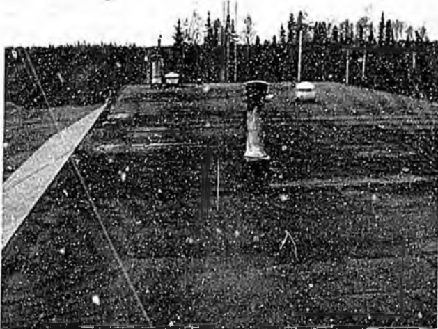
Photo No. 9 – View showing extent of recent repairs to roof membrane, in vicinity of furnace chimney. Dark areas were coated with repair product.
