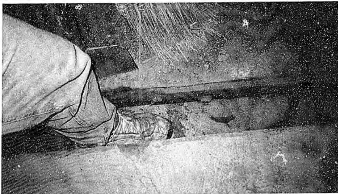
Photograph Eight: Floor slab separation and settlement.
